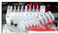
Control Terminal Block
