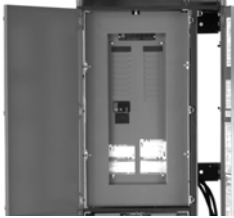
Distribution Panelboard in an MCC
