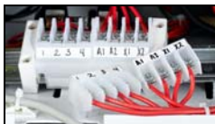
Control Terminal Block
