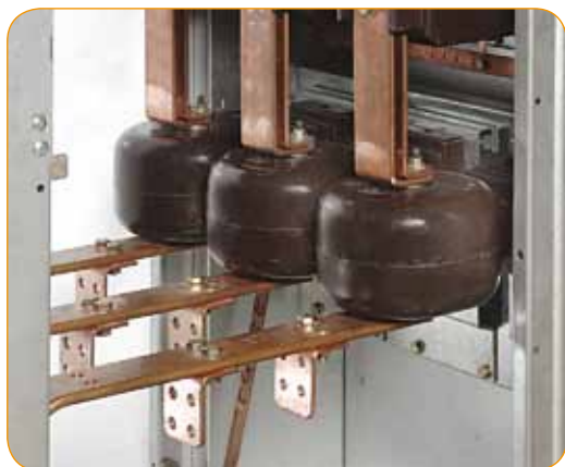
LPCT in cubicle
