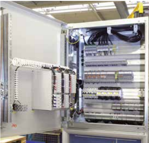
Low Voltage cabinet
