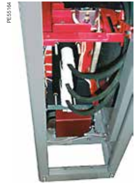
Floor cable entry
