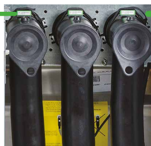
TH110 mounted on cable termination
