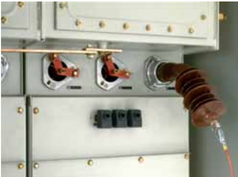
High-voltage cable test (1-phase) via test adapters mounted on the rear
