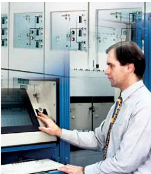
IMOS Monitoring and Operating System
