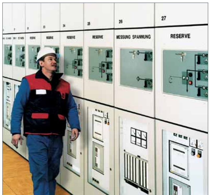
Front view of a double busbar switchgear WSB with operator
