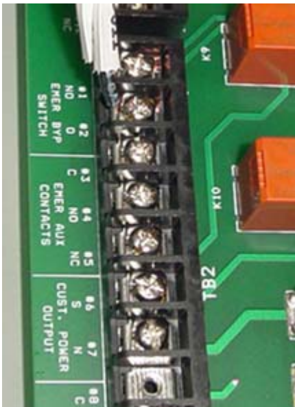
Figure 17: TCB Bypass Input (Terminal TB2—Terminal Points 1 and 2)
