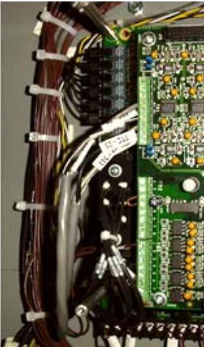
Figure 12: Fiber Optic Connections
